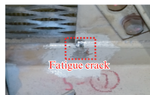
(a) Fatigue crack in crane structure
